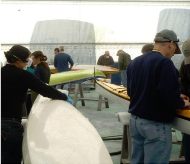
Kayak Fiberglass Repair Day, Annapolis Harbor Boat Yard photo by Anicca Jensen
